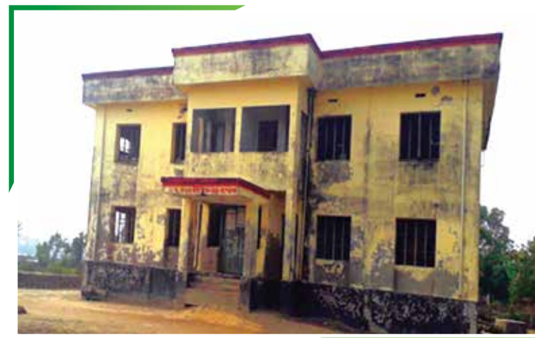
Figure 7: Damaged community clinic and connecting road by tidal surge and cyclone. Photo source: Field visit, December 2022, Shaymnagar, Satkhira.
