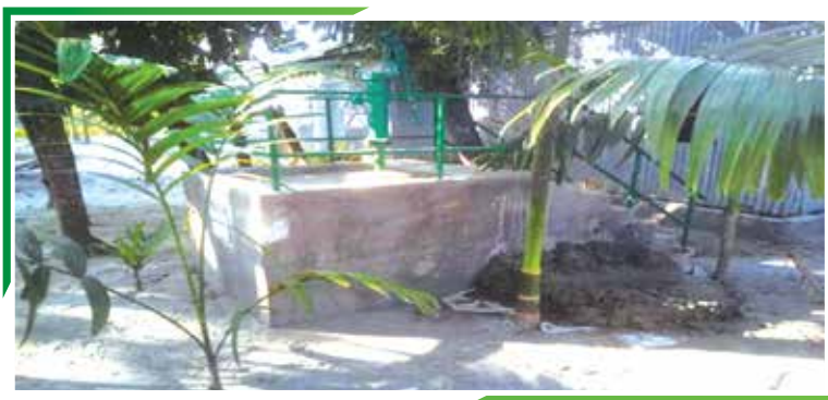
Figure 16: Installing tube well on high elevated place in char area. Photo source: Field visit, November 2022, Phulchari, Gaibandha.
